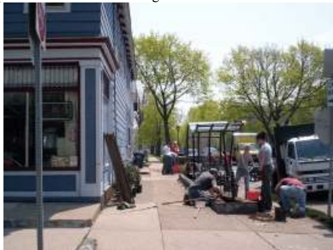
U. B. Students work to install new plantings at the bus shelter on Plymouth Avenue at Pennsylvania Street. Courtesy of Dan Greenway.
